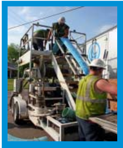
Resin-impregnated felt tube was shipped to the job site and inverted into existing manholes.
