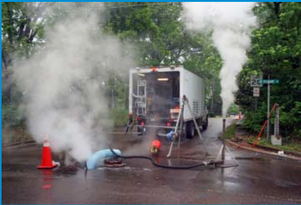
For some insertions, steam was introduced to bring the resin to its cure temperature.
