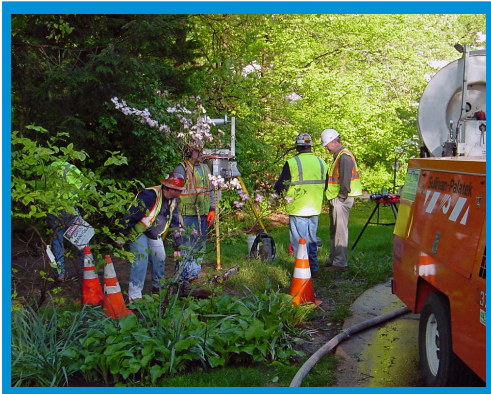
Insituform crews minimized disruption by using existing manholes for CIPP liner insertions.
