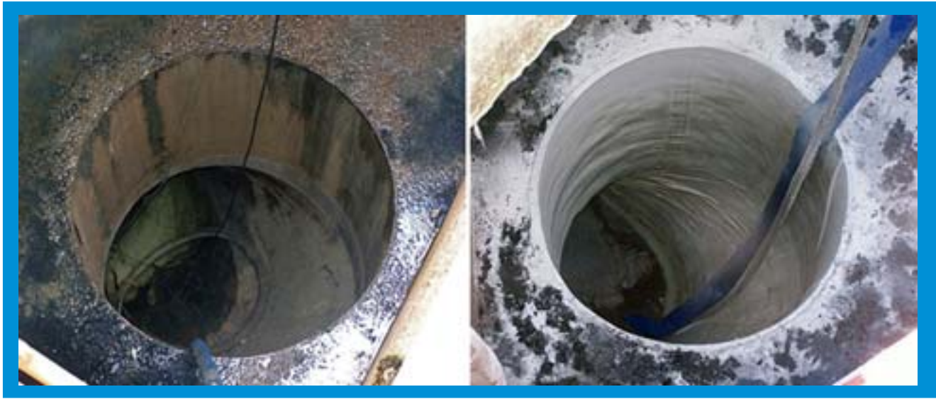
After the splitter box discharges were cleaned and prepared (left), they were lined with CIPP (right) and sealed.
