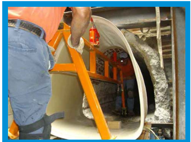
The original concrete pipe was in danger of failure because much of its protective tile liner was missing.
