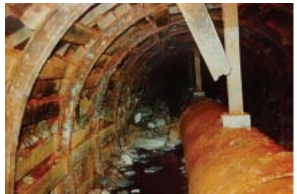
Waste water from breached carrier pipes escaped into the tunnels' annular space and created conditions that corroded the steel ribs. Eventually the wood lagging came loose and caused the marl behind it to spall. Photo courtesy of Charleston Water System.
