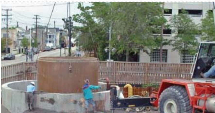
A 12-ft (3.6-m)-high, 10-ft (3-m)-diameter cast polymer composite section of a vortex drop shaft liner is lowered into place. Photo courtesy of U.S. Composite Pipe.
