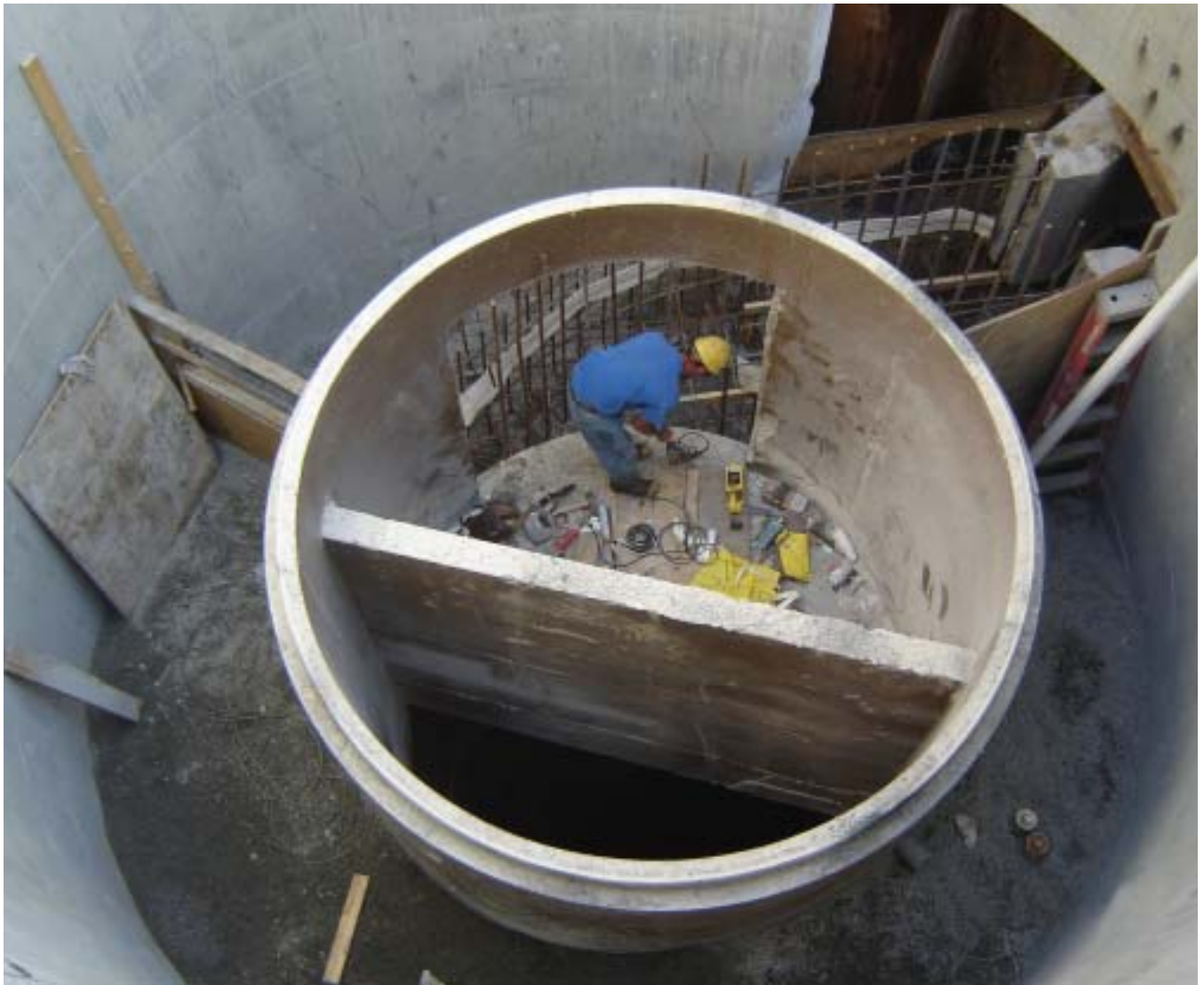
Shown is the installation of the next to last section of a precast polymer concrete pipe shaft liner. Photo courtesy of Black & Veatch.
