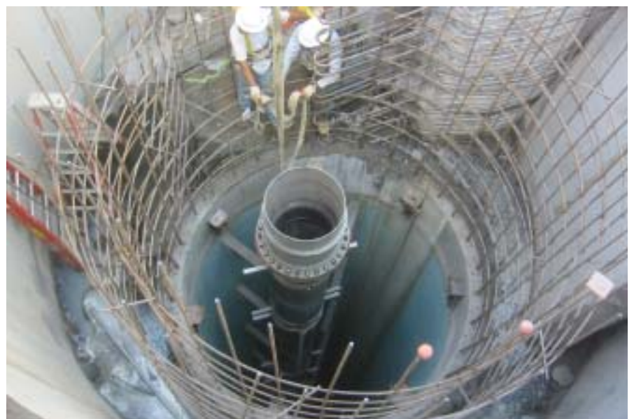
Workers construct a precast concrete pipe vortex drop shaft. This type of shaft consists of a HDPE drop pipe (center), and a SS wall pipe (the top portion of the center pipe) that forms the base of the scroll inlet. A 100% solids epoxy coating, 120 mils thick, is sprayed on the concrete interior of the shaft. Photo courtesy of Black & Veatch.
