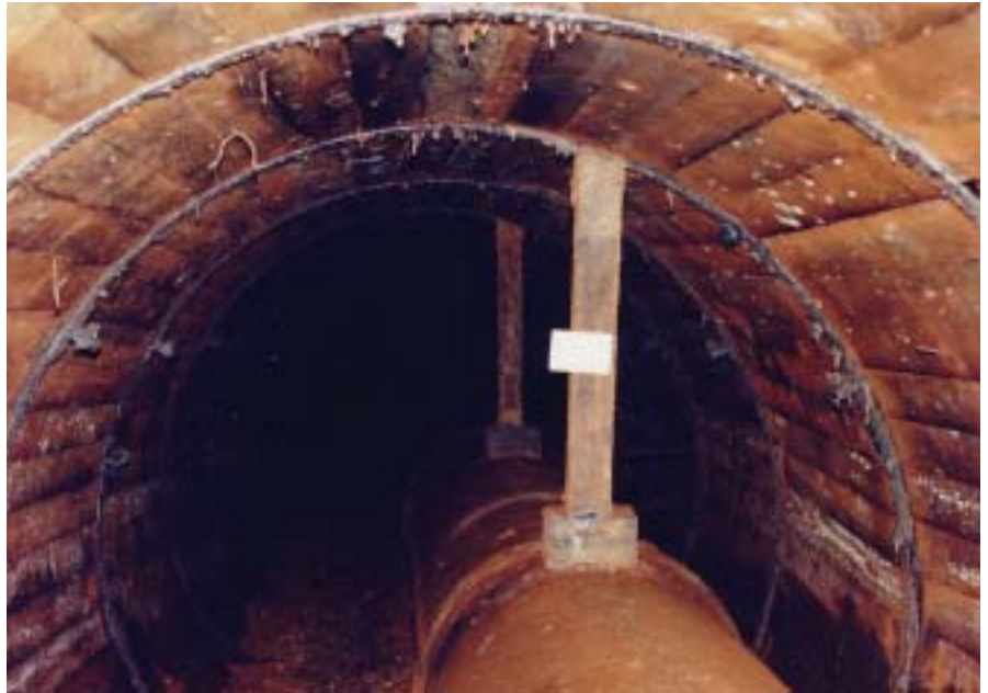
An intact section of the original tunnel. Photo courtesy of Charleston Water System.
