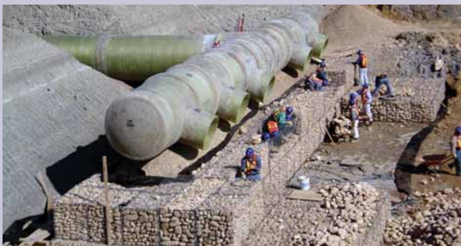
LNG re-gasification seawater intake diffuser.
