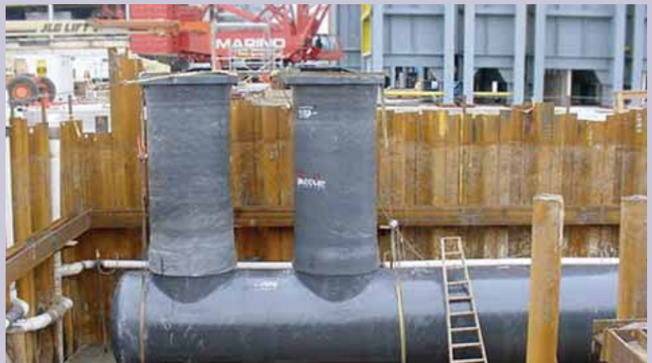
Header for power plant cooling water system.
