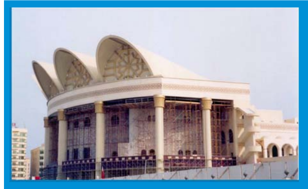
The half-cone-shaped vaults taper from 52.5 by 30 feet (16 by 9.25 meter) dimensions in front to 26.2 by 19.7 feet (8 by 6 meters) at the rear.
