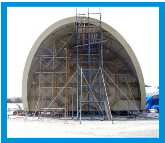
The front fascia with overhang was one of the six sections that were preassembled on the ground.
