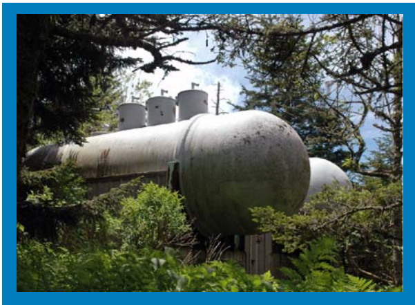
The two supply tanks provide a total capacity of 15,200 gallons.
