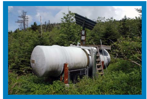
When available, solar power pumps water from the holding tank.
