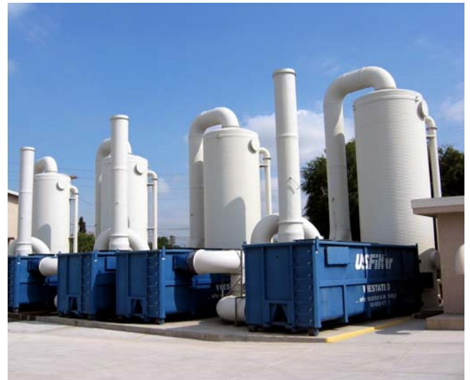
Air Chem Systems used Vipel® K022-C FR vinyl ester from AOC to manufacture four vertical scrubbers at a water treatment facility in Baldwin Park, California.
