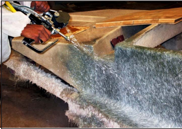
To effectively get around the tight corners of complex inner liners, skinning out is accomplished with a chopper gun.
