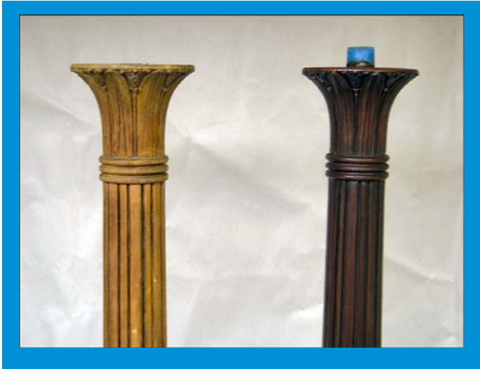
Details of the repaired original pole (left) are mimicked in the cast replica (the blue cap is the top of the cast-in-place wire chase).
