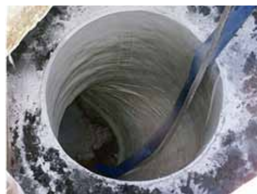
After the splitter box discharges were cleaned and prepared (left), they were lined with CIPP (right) and sealed.
