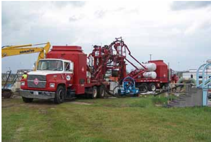
To minimize clarifier downtime, heated water from two boiler trucks accelerated resin cure.
