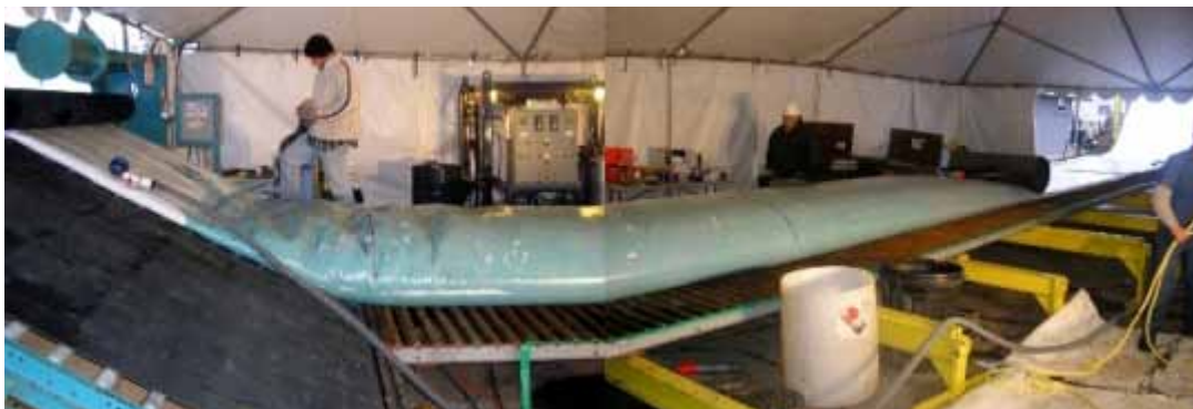
Felt tubing was impregnated inside a protective tent then conveyed out for inversion.
