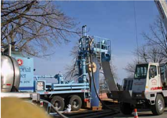
The project started in autumn before installation crews were challenged by the onslaught of a Green Bay winter.
