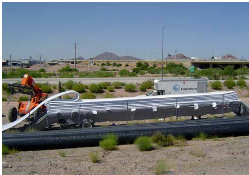
To repair large diameter concrete pipe, new liners were created by impregnating miles of Insituform® felt with Vipel® resin. (Image is used courtesy of Insituform Technologies, Inc.)
