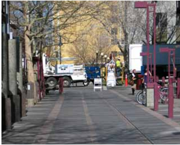
Trenchless technology for downtown Reno prevented disruptions to the city's busy convention trade.
