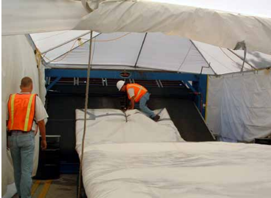
Including large diameter over-the-hole insertions, Reynolds Inliner has rehabilitated more than 76 miles of critical sewer pipe in the bustling Orlando, Florida, area.
