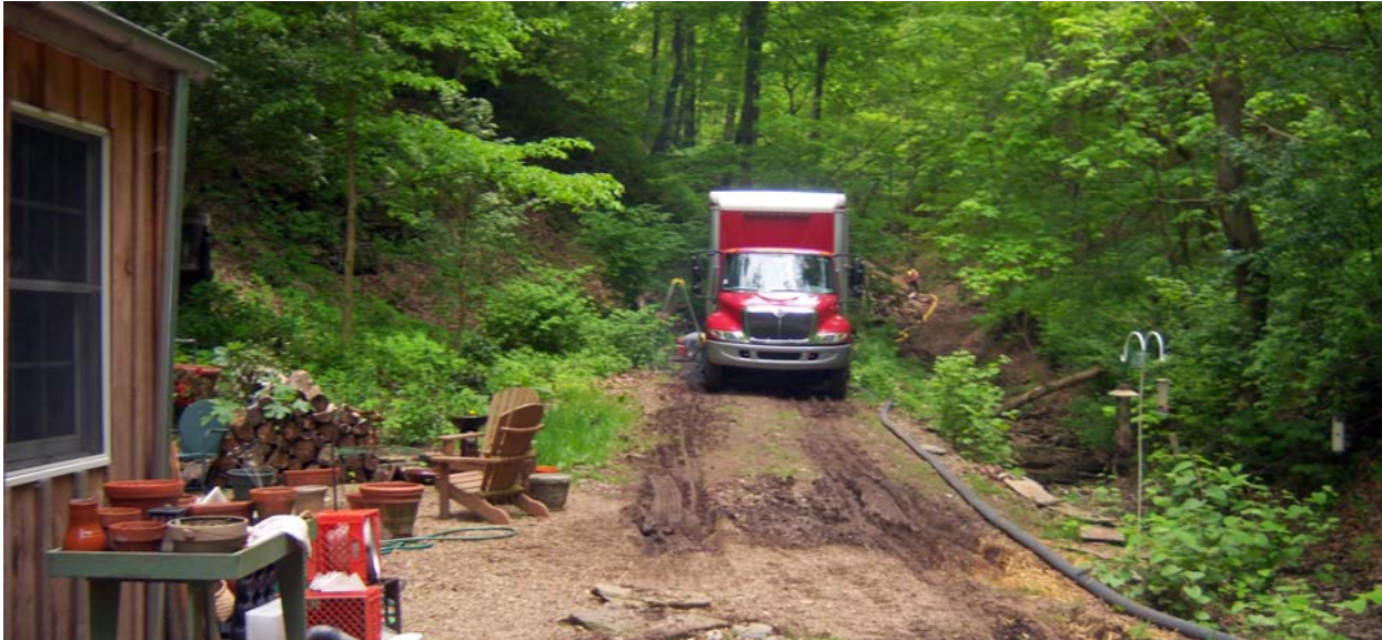
UV-cure technology was ideally suited for repairing pipe at the remote job site
