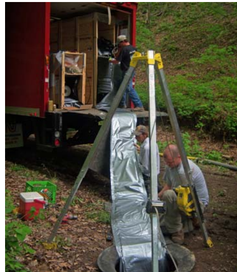
To eliminate excavation, the special Blue-Tek® slip sheet was guided into the host pipe through an existing manhole
