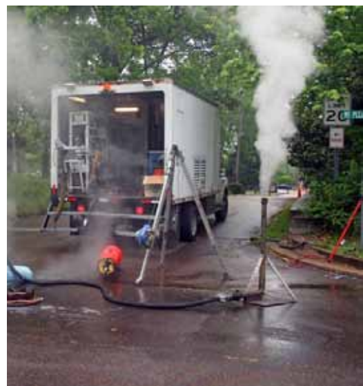
For some insertions, steam was introduced to bring the resin to its cure temperature.
