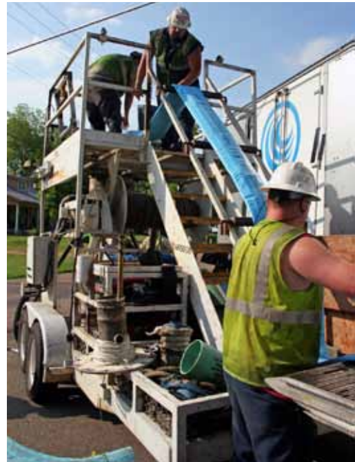
With trenchless CIPP upgrading the sewer's underground, the Southern charm on Collierville streets was not impacted.
