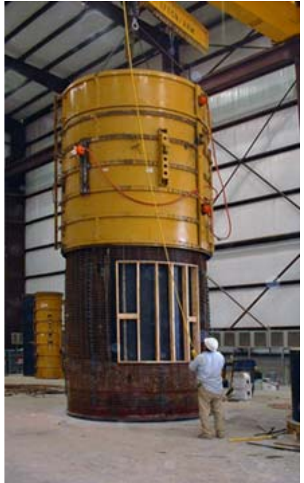
A worker sets the formwork for casting the 12-foot high vortex section.
