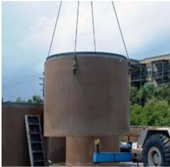
A worker sets the formwork for casting the 12-foot high vortex section.
