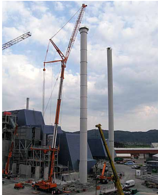
The composite liners were installed in a combined steel housing that was shipped to the plant site.
