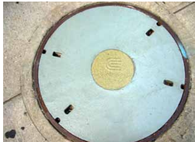
An installed hybrid cover prevents burns and branding.
