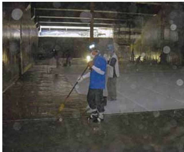
More than 40,000 square feet (3,700 square meters) of concrete surface were rehabilitated and strengthened.
