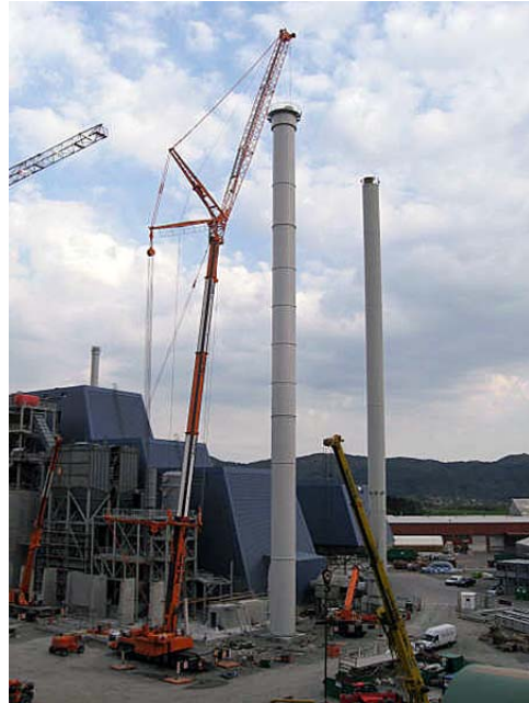
The composite liners were installed in a combined steel housing that was shipped to the plant site.
