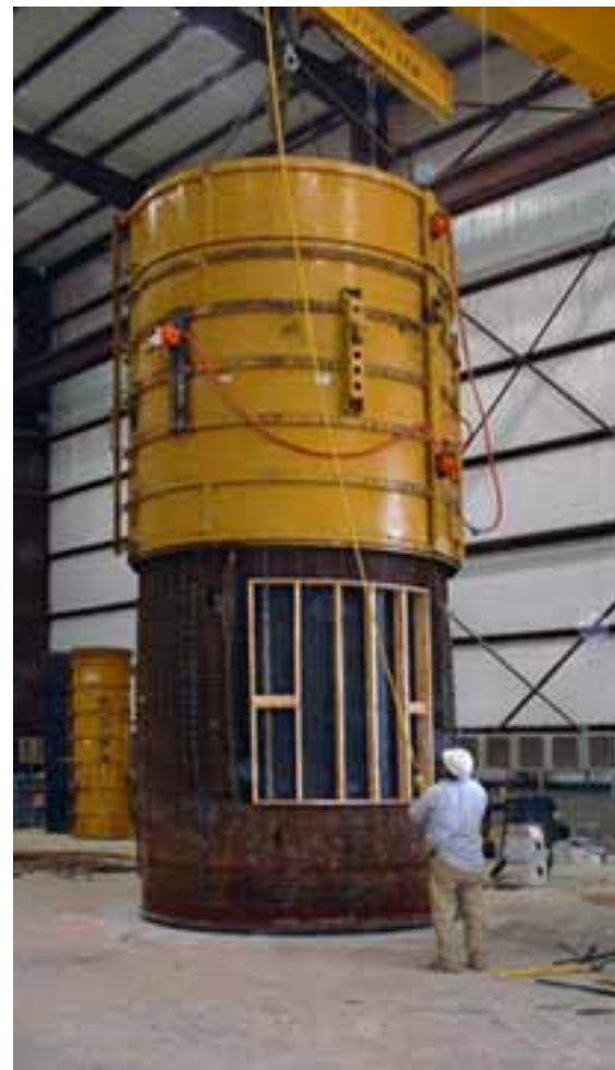
A worker sets the formwork for casting the 12-foot high vortex section.
