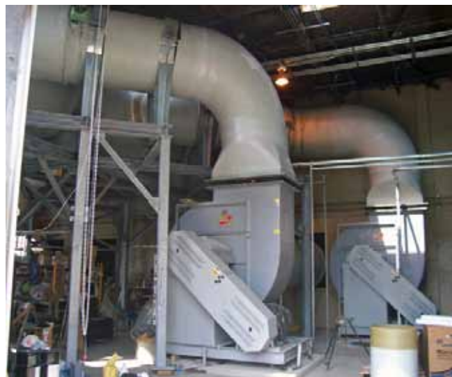
Composite ducting moves air toward the stacks.
