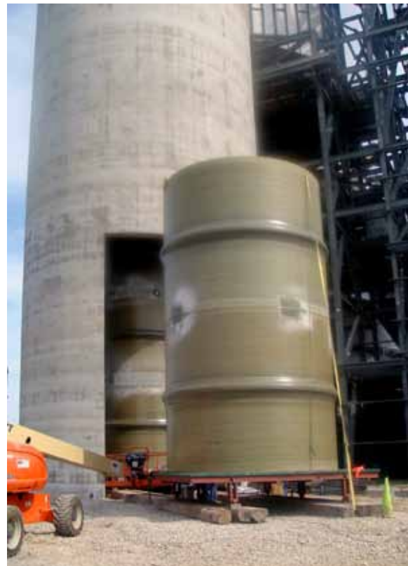
The composite cans were installed into the chimney to form a heat- and corrosion-resistant liner.
