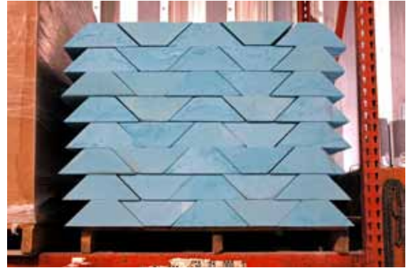
Pre-cut foam was integrated into the circumference of each section to help form exterior structural ribs that help support the liner.
