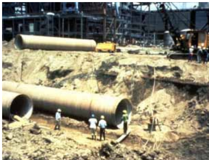
The light weight of the composite versus steel facilitated installation. Composite components in underground and aboveground sections are in very good condition after decades of use.
