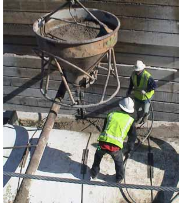
Concrete grout was poured in the space between the pipe and trench wall.
