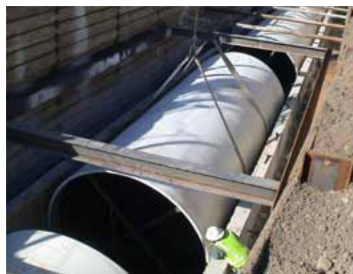
The 28-foot pipe sections were lowered through a 29-foot wide "window" then rolled into place.
