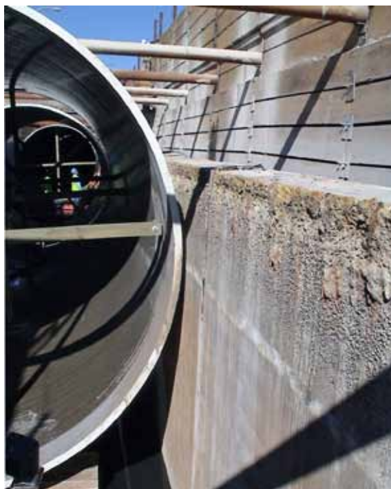
Belco custom-designed the pipe to fit precisely into the "trench" created by removing the damaged portion of the existing concrete culvert.
