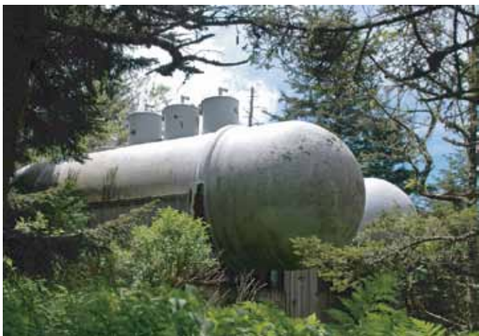
The two supply tanks provide a total capacity of 15,200 gallons.
