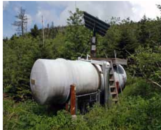
When available, solar power pumps water from the holding tank.
