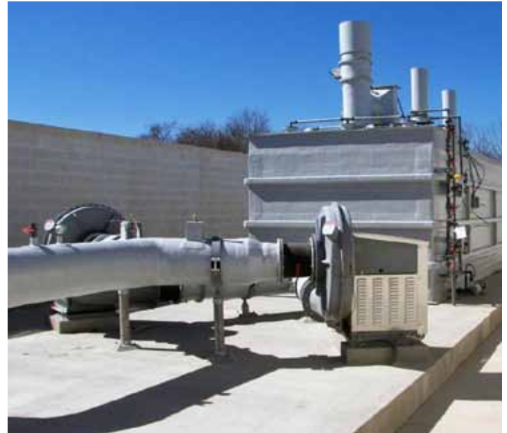
Vipel® technology helps the composite components resist the highly acidic nature of the odor control system by Bay Products, Inc.
