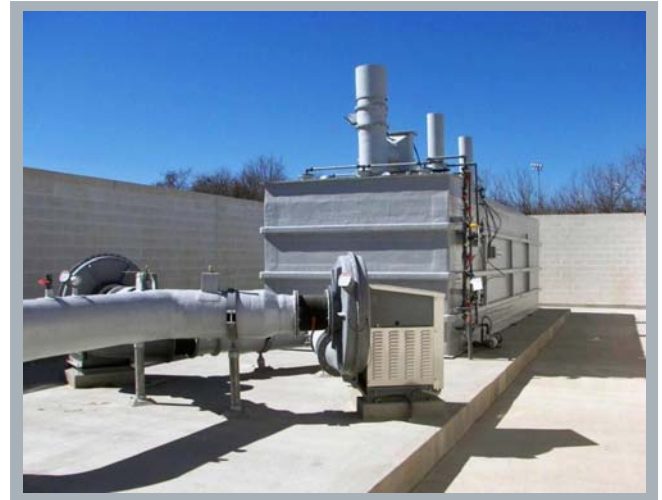
Vipel® technology helps the composite components resist the highly acidic nature of the odor control system by Bay Products, Inc.
