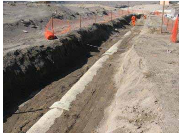
The project to expand the potable water supply for Arequipa City uses 9.8 kilometers (6.1 miles) of composite pipe.
