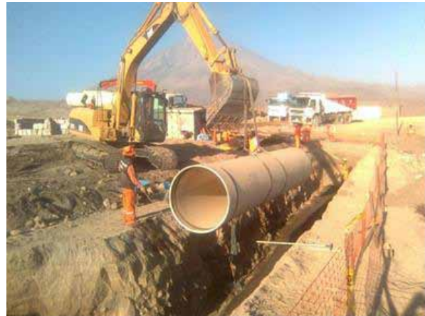
The lightweight of Flowtite™ composite pipe allowed the pipe to be installed without the use of heavy cranes.
