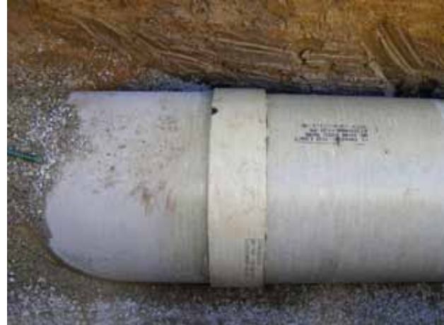
Stand-offs (white bands around the cylinder) allowed the pipe to be installed through existing iron drainage channels without having to excavate the channels.
