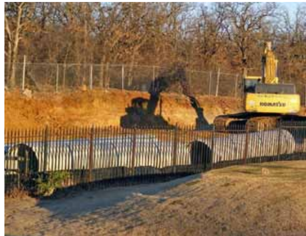
The project needed 4,700 feet (1,433 meters) of Flowtite® composite pipe made with optimized Vipel® resin technology.
