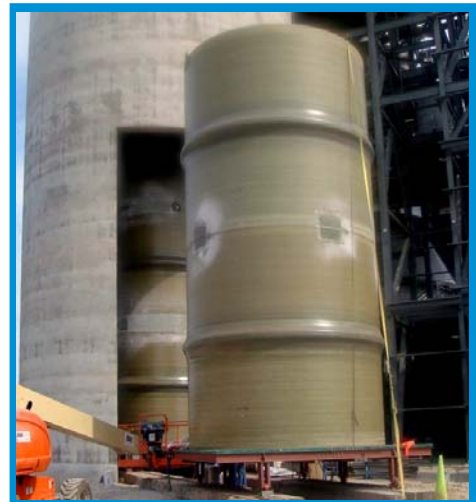
The composite cans were installed into the chimney to form a heat- and corrosion-resistant liner.
