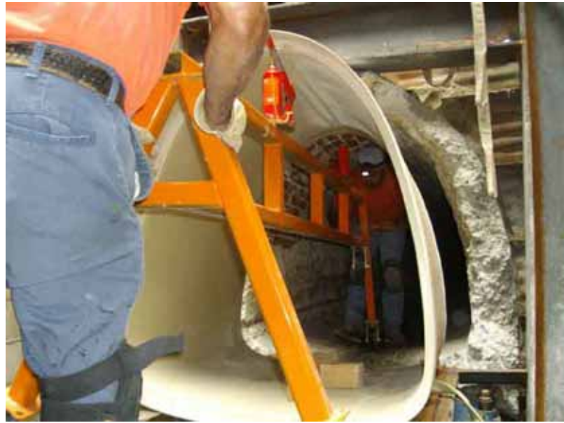
The original concrete pipe was in danger of failure because much of its protective tile liner was missing.
