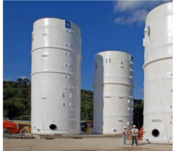
Tank sections manufactured under ASME-certified conditions were assembled at a riverside site.
