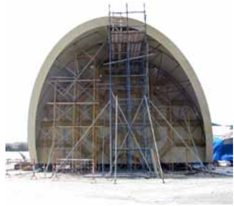
The front fascia with overhang was one of the six sections that were preassembled on the ground.
