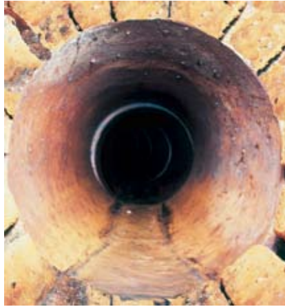
Before repair with Vipel® technology
