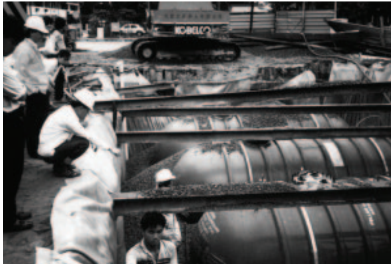
Figure 6. In 1994, composite underground storage tanks are installed at Mobil service stations in Singapore.
