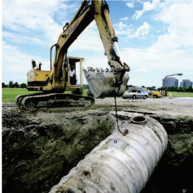
Figure 4. UL-1, the first composite tank to earn a UL listing, is unearthed after more than 25 years of service.
