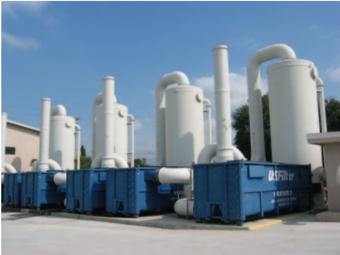
Figure 1. Composites towers and ancillary equipment for scrubbers at a water treatment facility in Baldwin Park, CA, USA.
