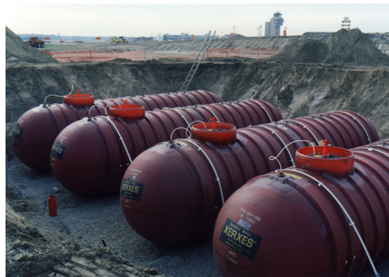
Fuel storage tanks
