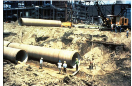
The light weight of the composite versus steel facilitated installation. Composite components in underground and aboveground sections are in very good condition after decades of use.
